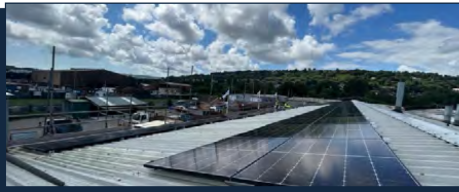
Here's our panels hard at work!
